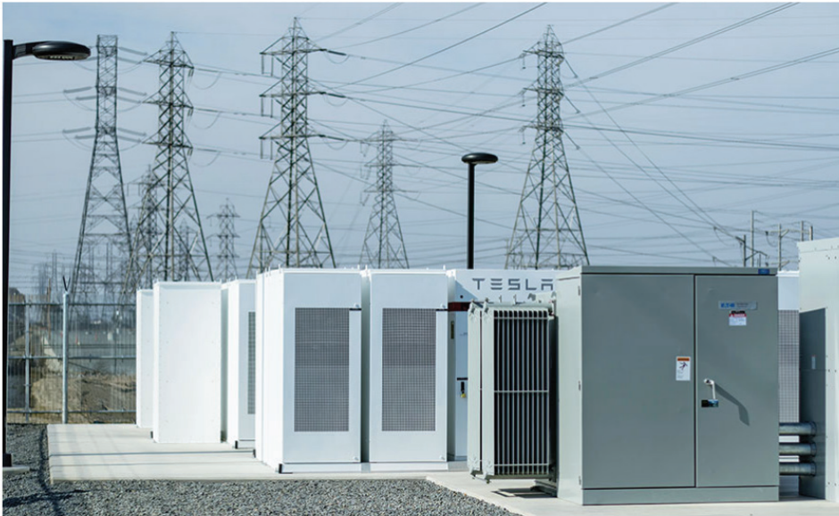
Southern California Edison's Mira Loma Battery Storage Facility uses Tesla-manufactured lithium-ion batteries to bank for later use renewable energy generated during low-demand periods.
